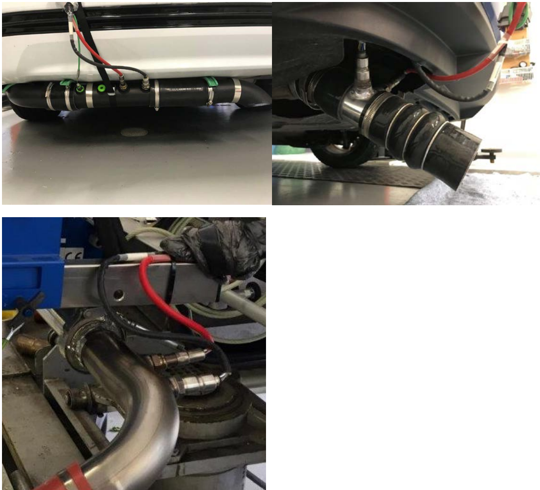
Figure 30. Example of installation of MiniPems. Red cable show the CO/CO 2 -sensor and black NO x and lambda sensor
